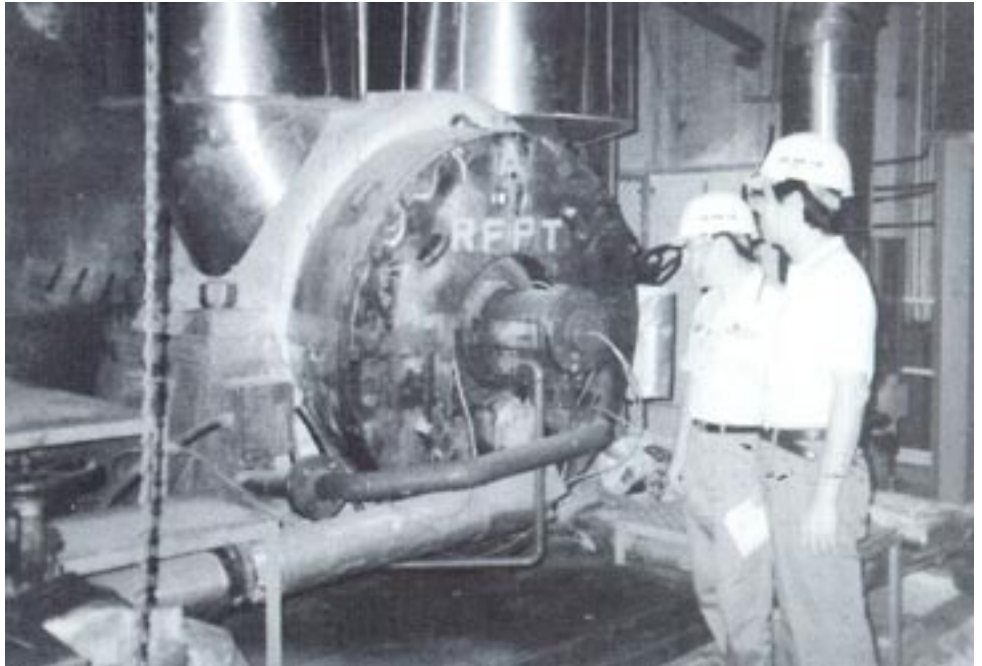
The Kuosheng 2 reactor feedwater pump.
